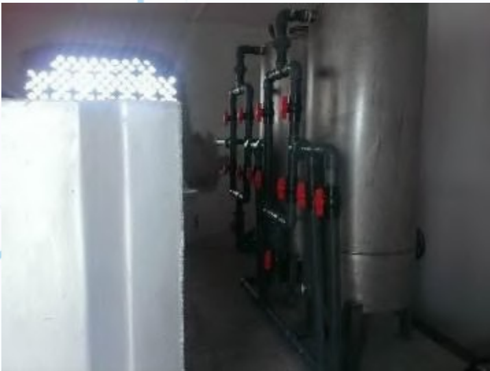
TRADITIONAL WATER TREATMENT INSTALLATION
