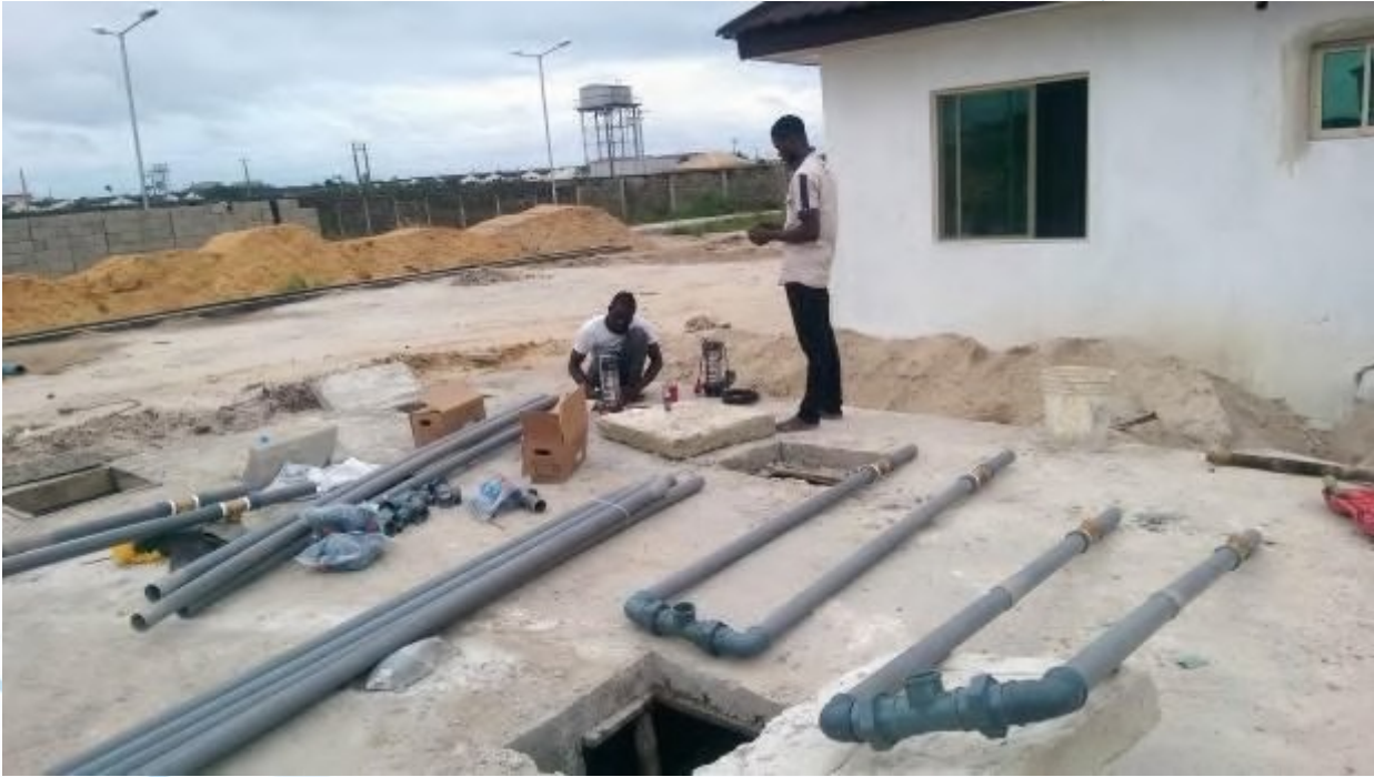
EXTENDED AERATION SEWAGE TREATMENT INSTALLATION
